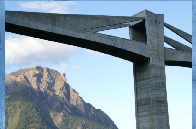
Fig. 2: The Ganter bridge with a span of 678 m is affected by ASR.
