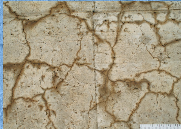
Fig. 1: ASR-typical crack pattern with dark linings of extruding reaction products.
